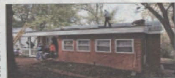
Volunteers Elizabeth Anderson and Kelly Yellonick, TRD, paint inside Healey's house. ABOVE, volunteers and local business sponsors work on, in and around Healey's home.
